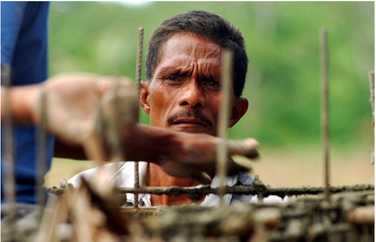
Shelter construction may provide an opportunity for people to learn new skills. Photo: Australian Red Cross/Mario Jonny dos Santos
